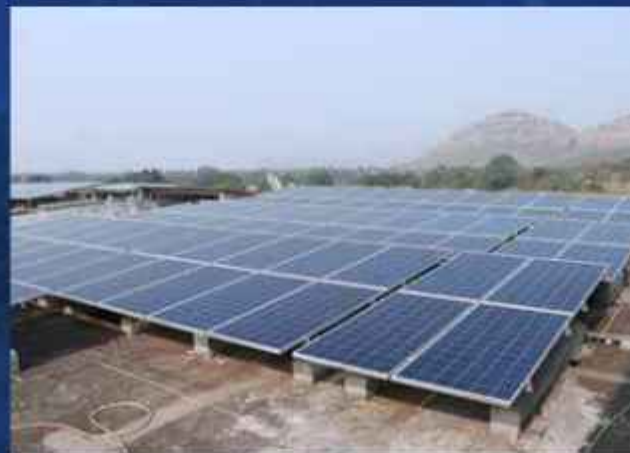
Solar Energy Plant
