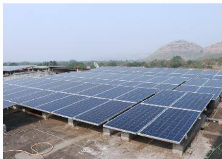
Solar Energy Plant
