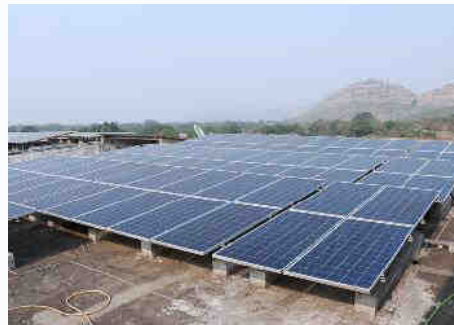
Solar Energy Plant
